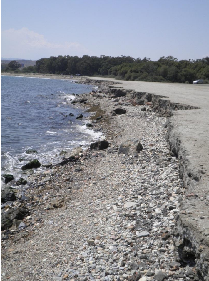
Figure 4.4. Front of erosion located at Quitapellejos beach. Note that coarse grain size instead of sand beach is nowadays presented in this area.
